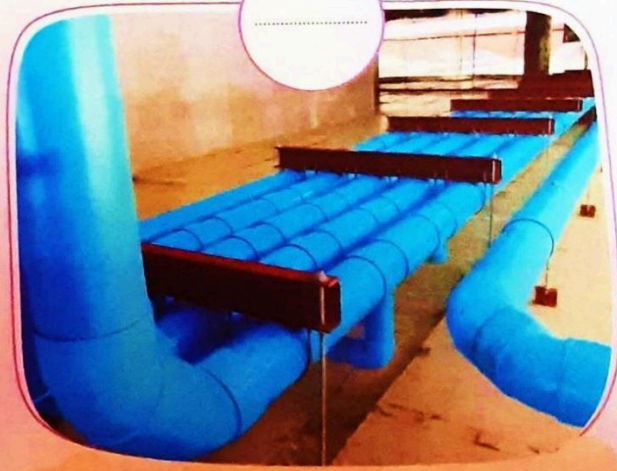
Clean water goes from filtration station to pipes.
